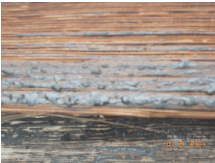
Suspect asbestos-containing material H-13-N-TR01. The tar material is non-detect for asbestos.
